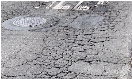
Impervious, deteriorating surface
