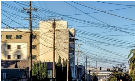
Dangerous overhead wires
